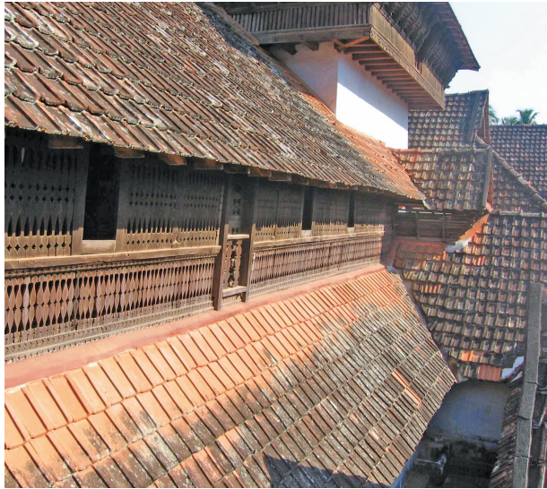
The roof comes down very low protecting the walls from the sun; Thekke Kottaram, a building which is part of the Padmanabhapuram complex.
